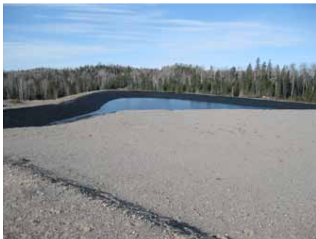
Photo 2. Ore pad and containment pond at Shebandowan West project site
